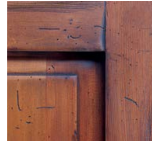
EXTRA HEAVY DISTRESS Heavy distress with deeper gouges, marks and scars. Small sections are wirebrushed and torched.
